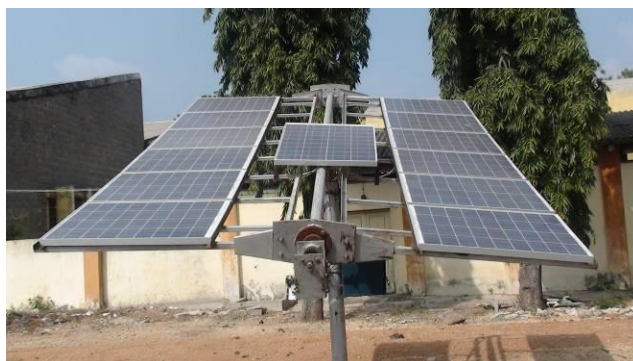
A view of the solar pumping unit established at UAS campus
